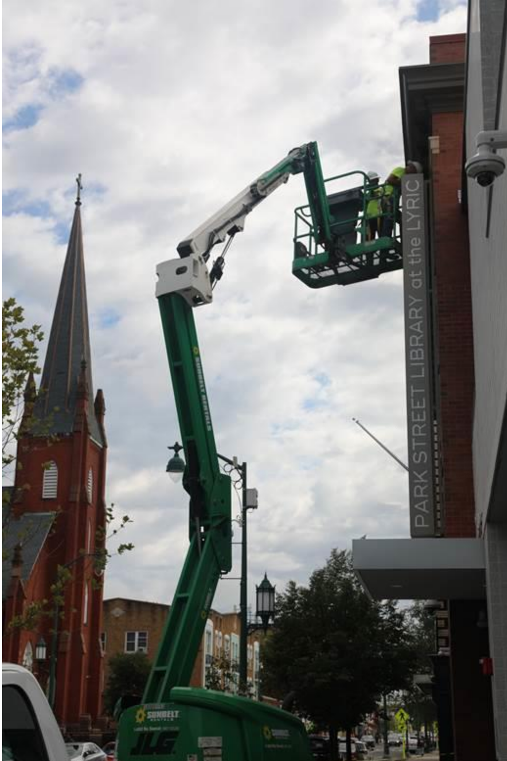
A sign is installed at the new Park Street Library @ The Lyric on Thursday, Sept. 16, 2021, in Hartford. The new library, which is nearing completion and will be the Hartford Public Library's largest branch location, will open its doors to the public for a community celebration on Oct. 2. (Photo by Russell Blair / Hartford Public Library)
